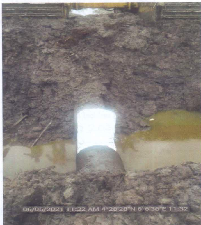
FIG.2 SHOWING SPILL POINT (AFTER REPAIR)
