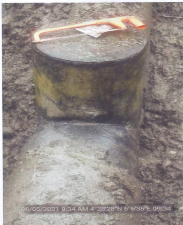
FIG. 1 SHOWING SPILL POINT (BEFORE REPAIR)
